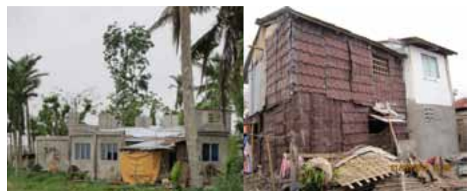
left photo: The second floor of a house made of concrete hollow blocks in Pan-Ay, Capiz was completely destroyed by typhoon Yolanda.
