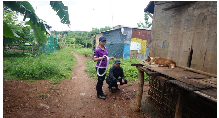
Ara learns how to properly stake a lot together with her fellow intern and schoolmate, Gab Gersaniba, during their visit in Masagana Angat resettlement area.
