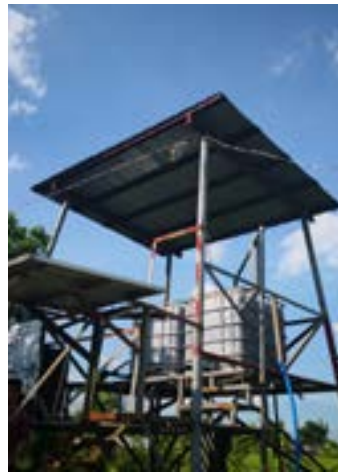
Solar-powered water pump supplying all the water requirements of Mangarita Farm.
